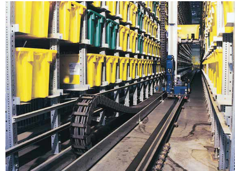
igus® steel guide trough used in a storage and retrieval equipment with series E2/000 and chainflex® cables
