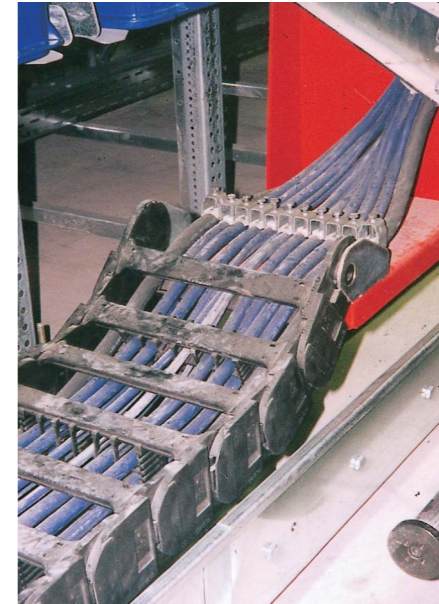
Example of lowered mounting height, in field operation
