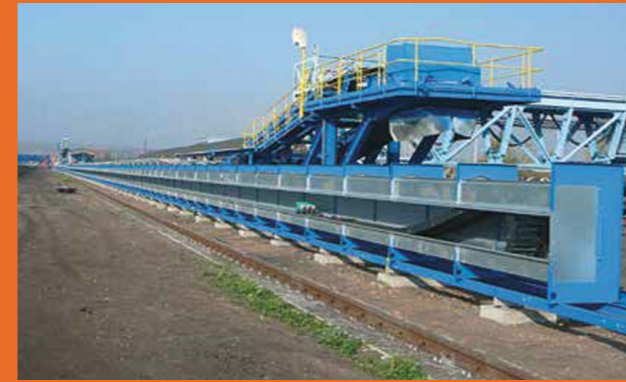
The worldwide longest e-chain travel of 615m with igus® rol e-chains® and chainflex® cables in a power plant
